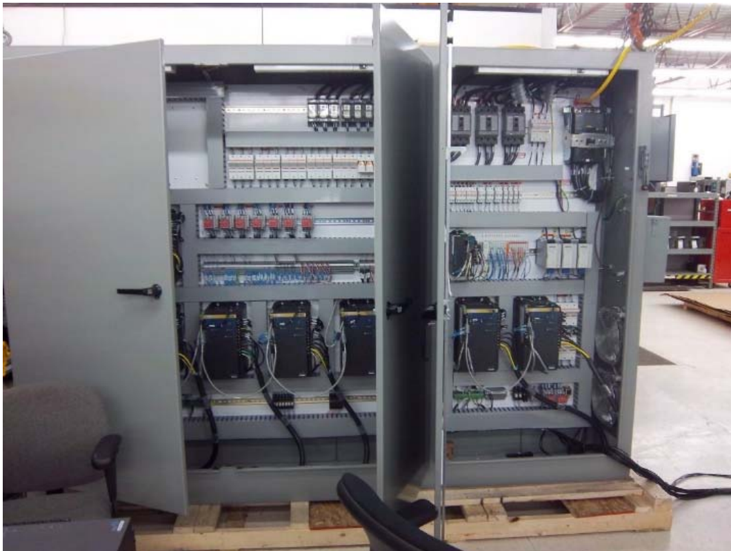
Figure 2: 9-Axis 50A/Drive Panel for NASA, installed in a converted CONEX Box, also designed by ORMEC
